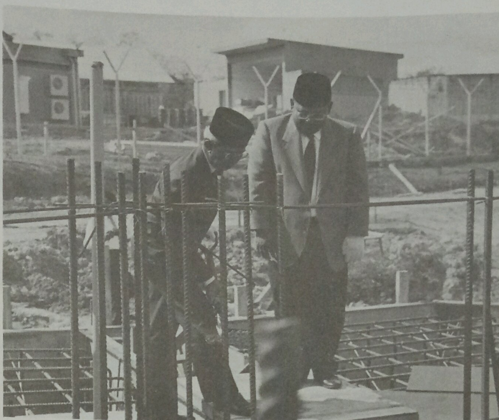
The Permanent Secretary of the Ministry of Communication, Dato Paduka Haji Awang Ahmad lays the foundation stone on the site of Brunei Darussalam's digital earth satellite station at Telisai in the Tutong district, while the Director of the Telecommunications Department, Dato Paduka Awang Haji Abdullah looks on.
